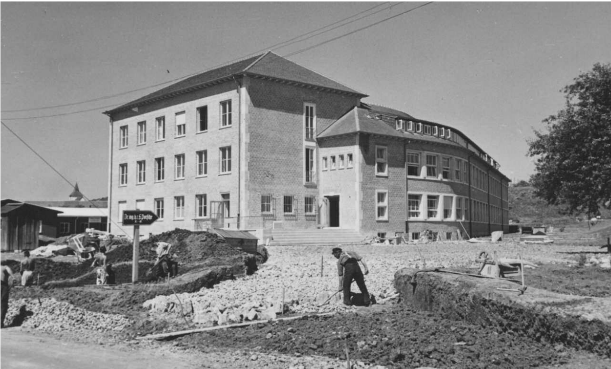
Plant 1 in 1938: The construction work has just been finished. Today, the “brick building” is a central component of the plant in Zuffenhausen
